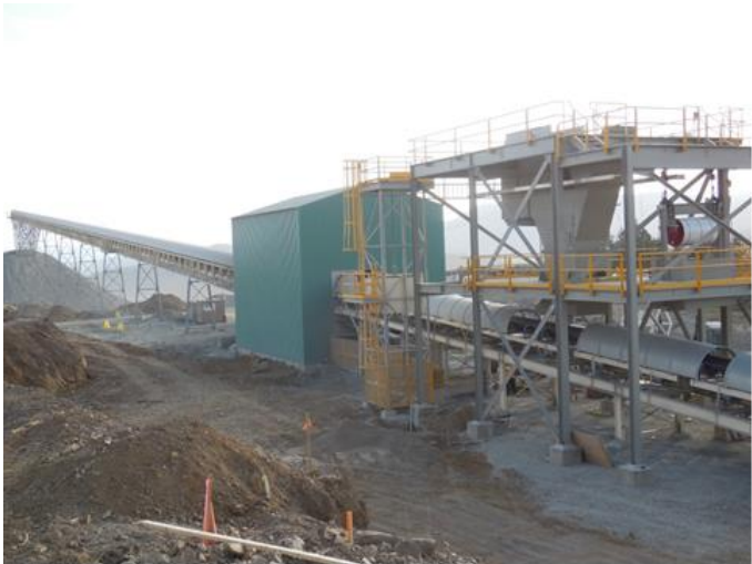
New Drive and Transfer Tower located on south side of drive house
