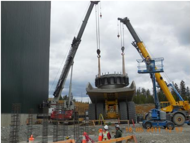
Loading Upper Main Frame into 240 ton haul truck in preparation for installation in Crusher Building
